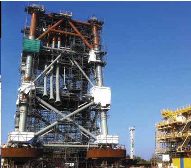
Fos-sur-Mer: scaffolding for the construction of modules for the "Anguille" offshore platform.
