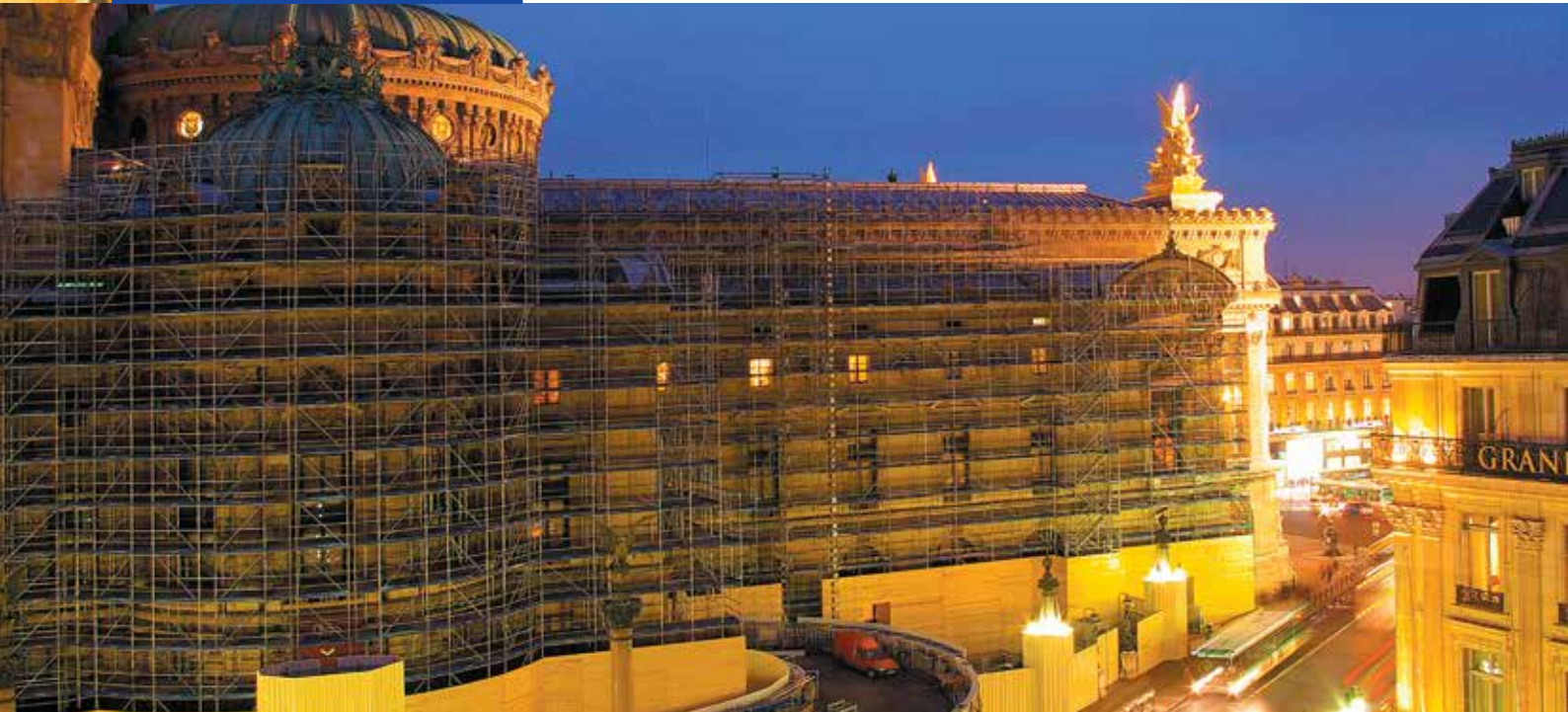
Paris, Opéra Garnier: scaffolding for the restoration of the west facade and cupola.
