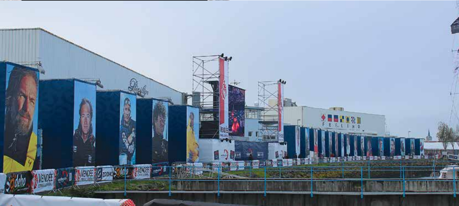
Les Sables-d'Olonne, Vendée Globe race: 180 m long scaffolding wall consisting of "totem towers" supporting the sailor's portraits.
