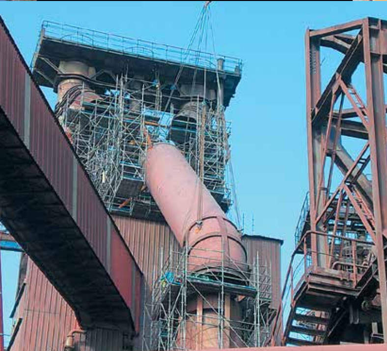
Arcelor Mittal Atlantique et Lorraine site: scaffolding for maintenance work on blast furnace No. 2.
