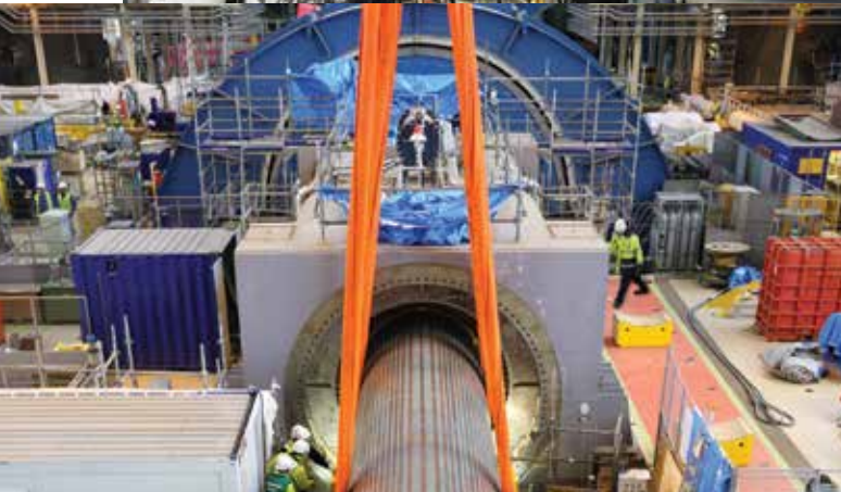
EPR, Flamanville: a huge amount of scaffolding and shoring has been supplied to this project since its inception.
