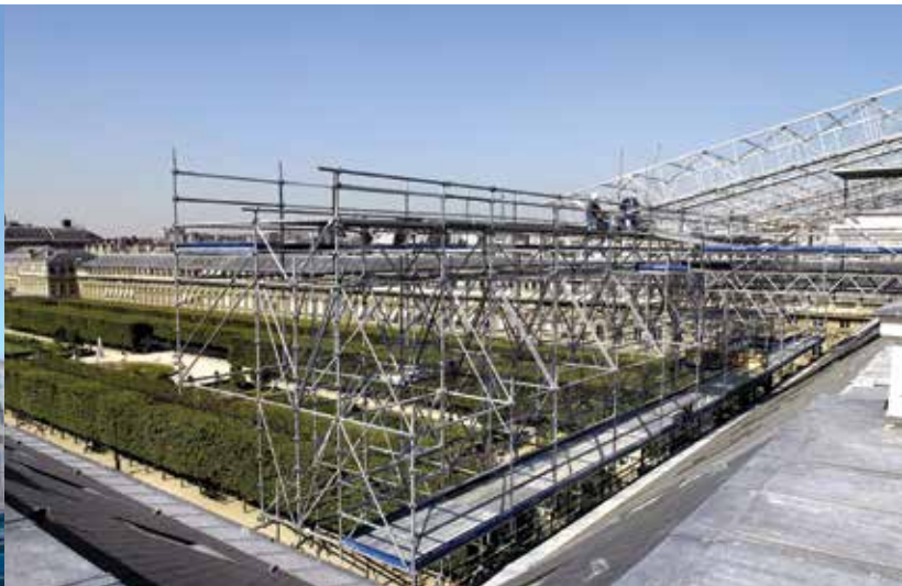
Paris, Palais Royal: temporary roof for renovation work to the headquarters of the Banque de France.
