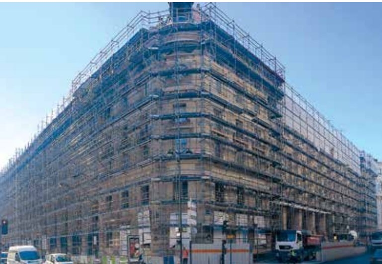
Paris, Louvre post office: 230 tonnes of Multicrab scaffolding for the 9200 m 2 of the building's four sides.
