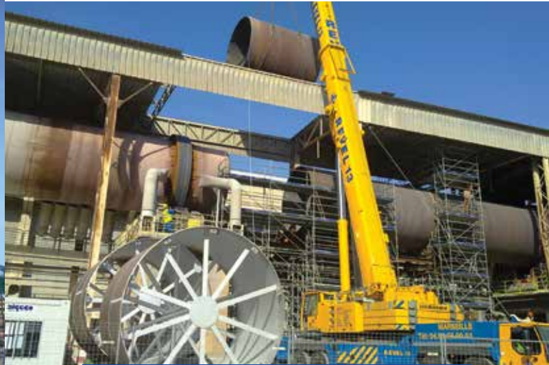
Ciments Lafarge: scaffolding and shoring for the replacement of a furnace shell.
