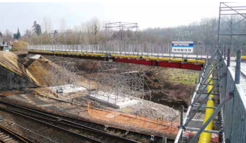
RN 21, between Limoges and Périgueux: temporary footbridge during reconstruction of the bridge over the railway.
